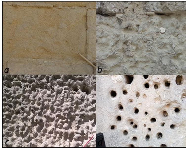
Figure 3 – Most frequent morphologies derived from loss of stone material in Gravina Calcarenite of the Matera Sassi: (a) roughening of lithoclastic calcarenite; (b) differential erosion of bioclastic calcarenite; (c) natural and anthropic perforations; (d) alveolization mixed to differential erosion.
