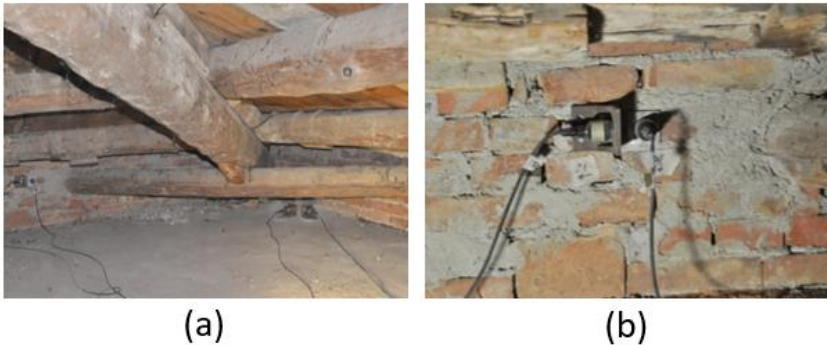
Figure 5.22. a) View of the installed sensors; b) detail of the sensor with the plate
