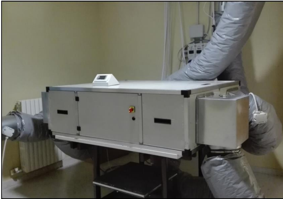
Figure 14: SIVeMeC installation and its connections with climatic rooms.
