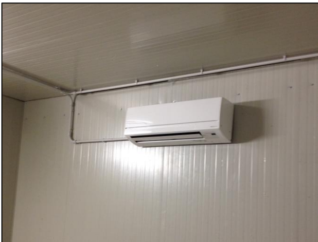
Figure 8: confined environment split unit.
