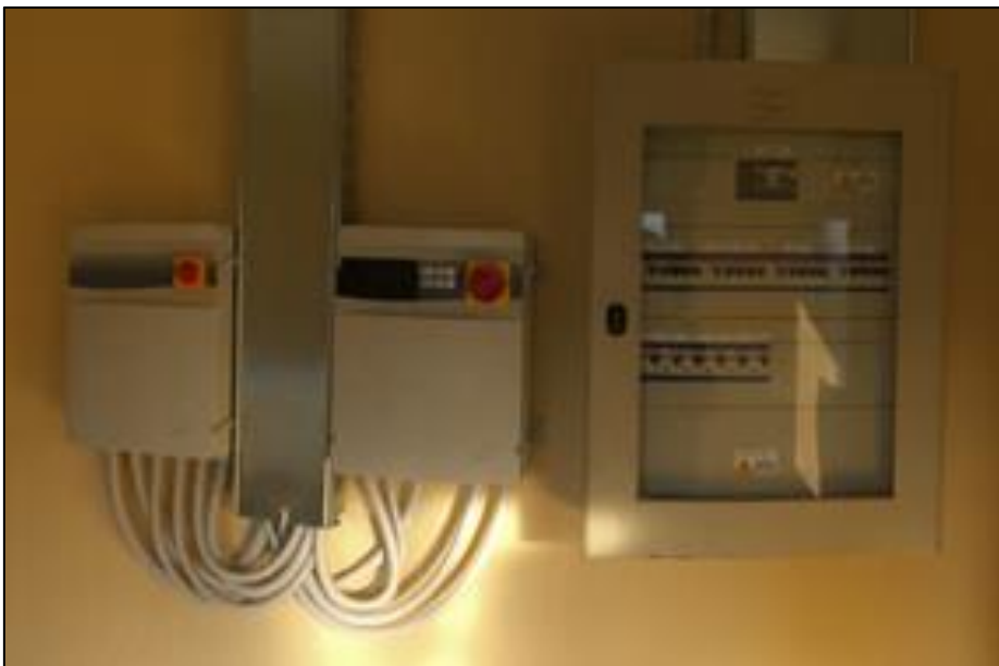
Figure 13: electric power panel and refrigeration plant panels.
