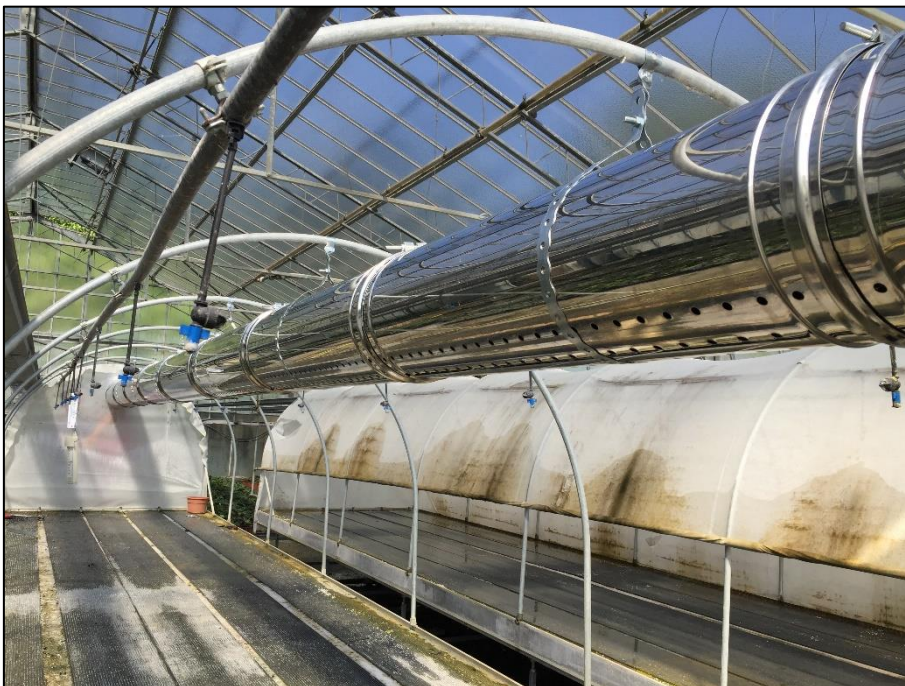
Figure 46: perforated duct for supply air distribution.
