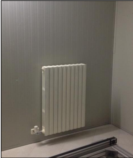
Figure 9: radiator with thermostatic valve.
