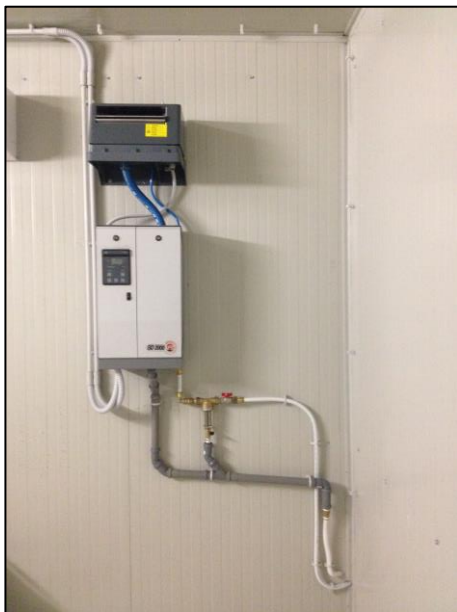
Figure 10: immersed electrodes humidifier in the confined environment.
