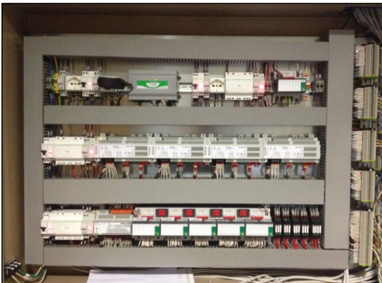
Figure 12: general control panel.
