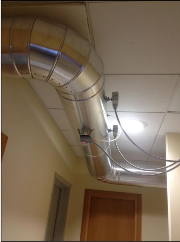
Figure 5: connection duct from external environment to the suction side of the system.
