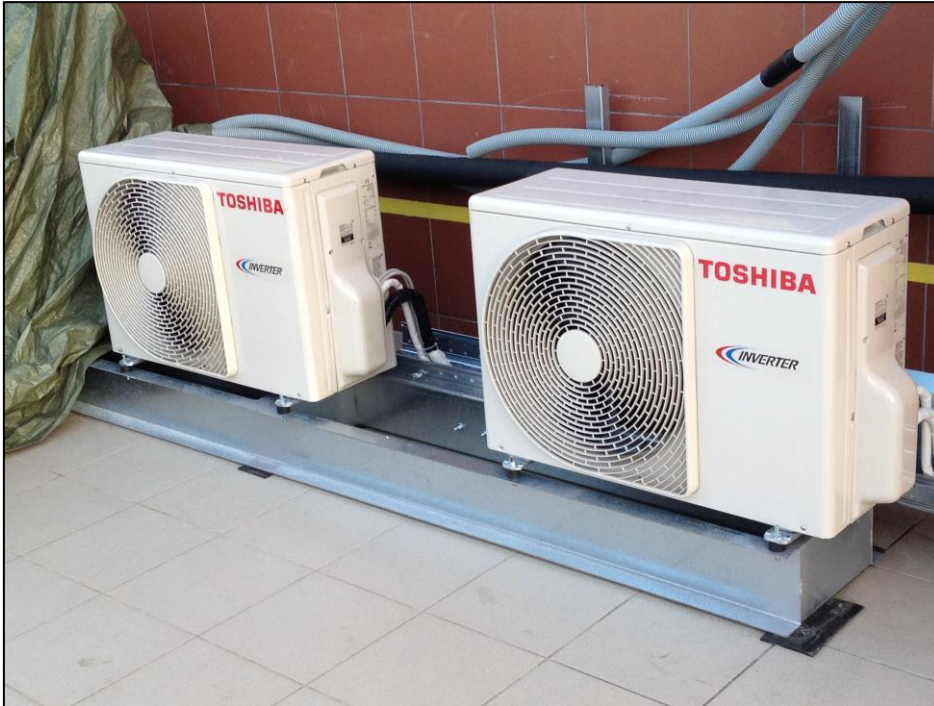
Figure 7: heat pump external units.
